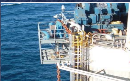
This compact chain jack has a holding capability of nearly twice that of adjacent mooring winches
